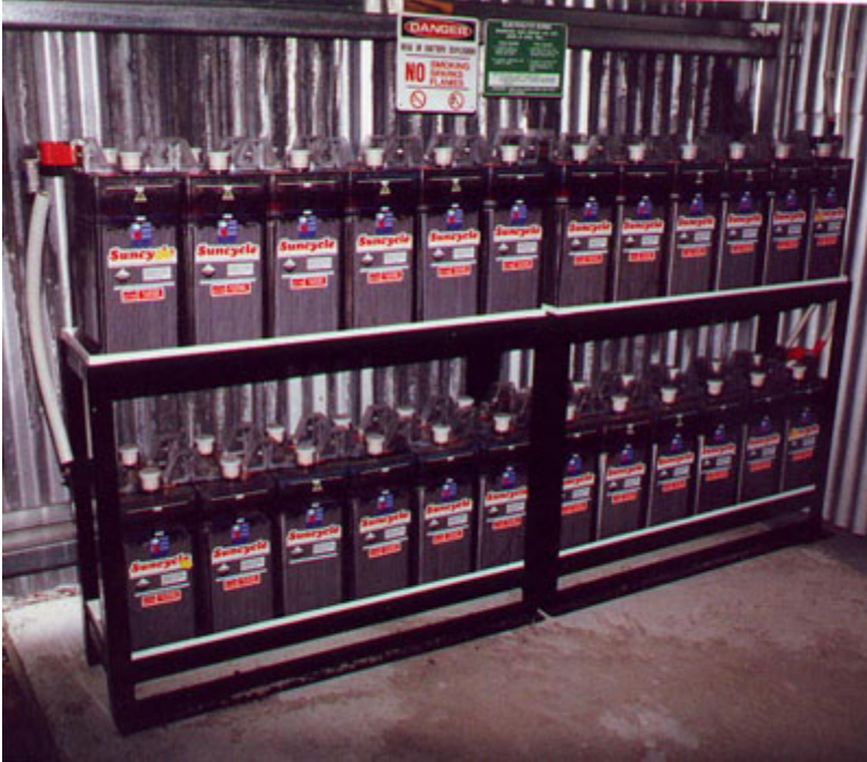
Figure 5. 48V DC Battery Bank (Photo courtesy of MUERI )
