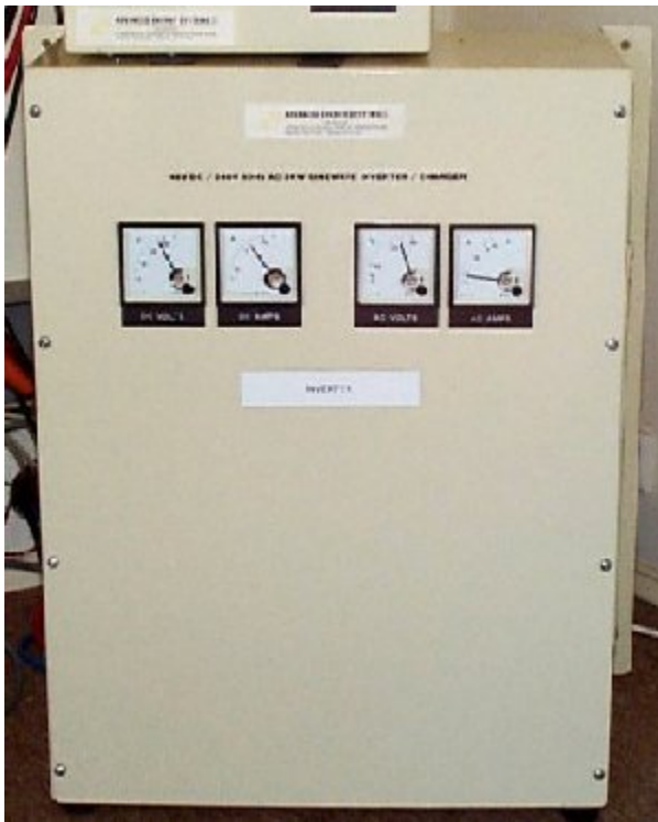
Figure 7 Photo of an inverter (Image courtesy of MUERI )
