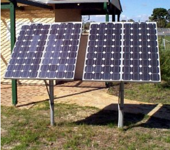
Figure 3 Small solar array (Image courtesy of ACRE )
